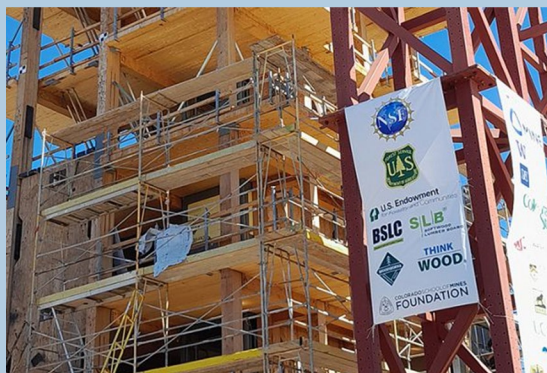
The 10-story mass timber building under construction on the shake table. Credit: Shiling Pei/Colorado School of Mines.
