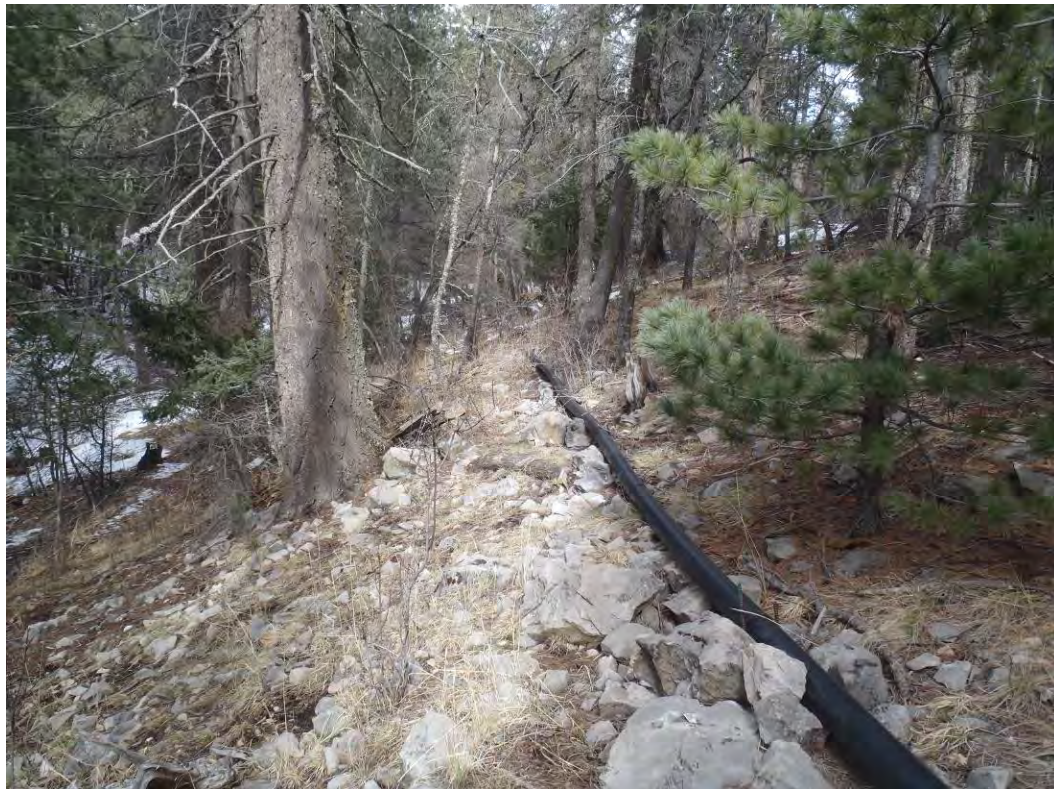
Photo 6: Wastewater discharge perforated piping facing northwest
