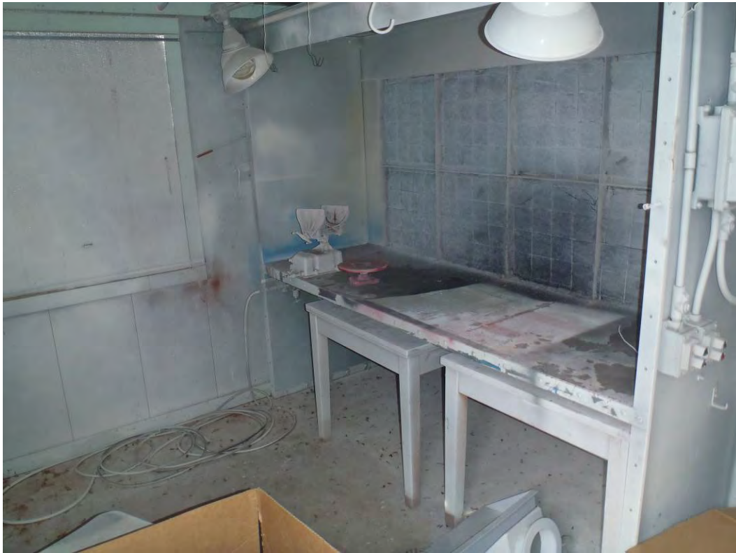
Photo 31: Inside paint booth
