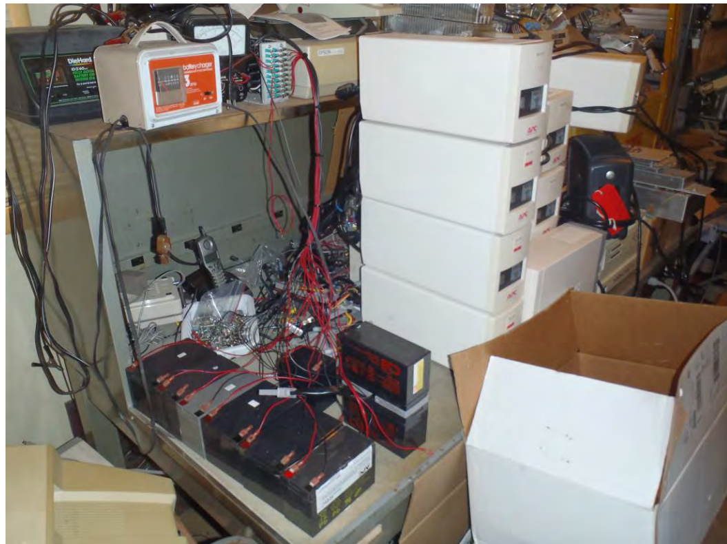
Photo 38: Battery charging area in main lab
