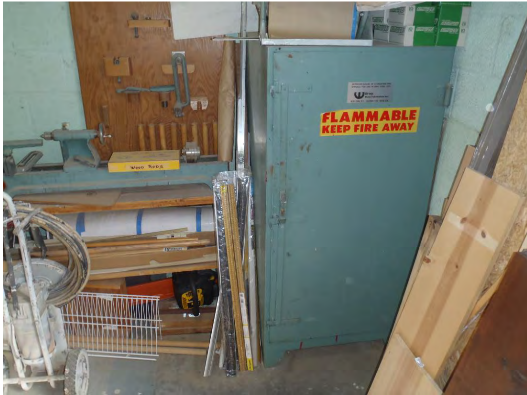
Photo 19: Flammable locker inside machine shop
