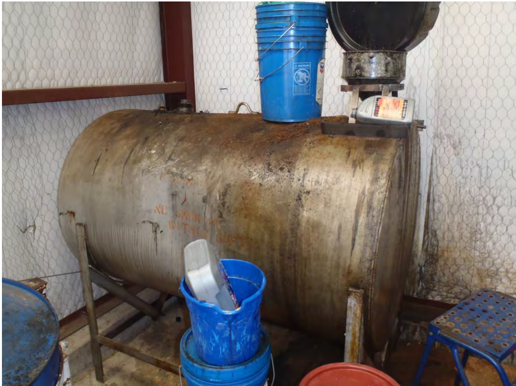
Photo 21: Used oil tank inside hazardous waste building
