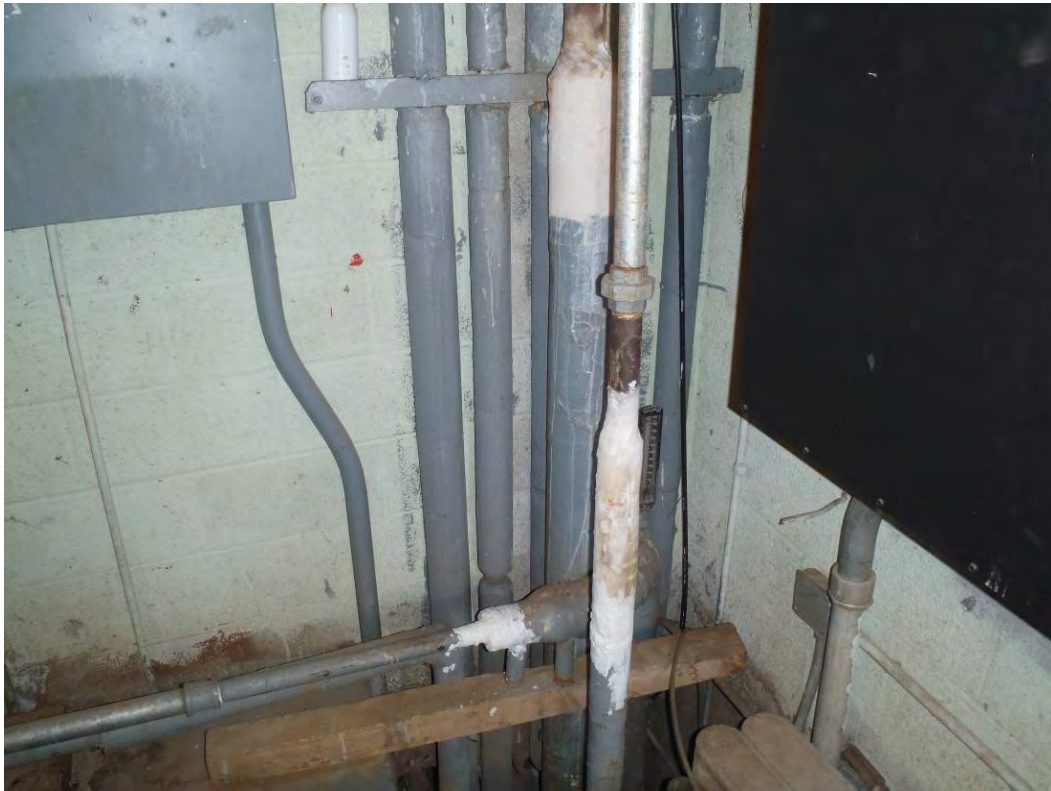
Photo 41: Suspected asbestos-containing material in main lab
