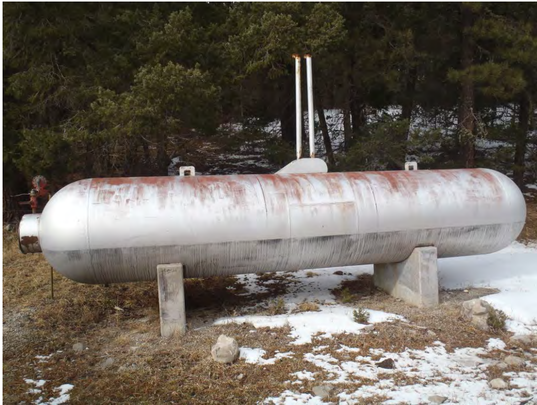
Photo 5: Propane tank at wastewater treatment facility facing north
