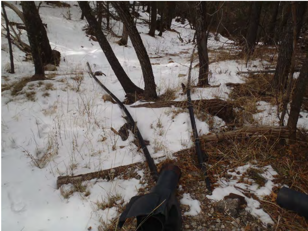
Photo 7: Wastewater discharge perforated piping facing west
