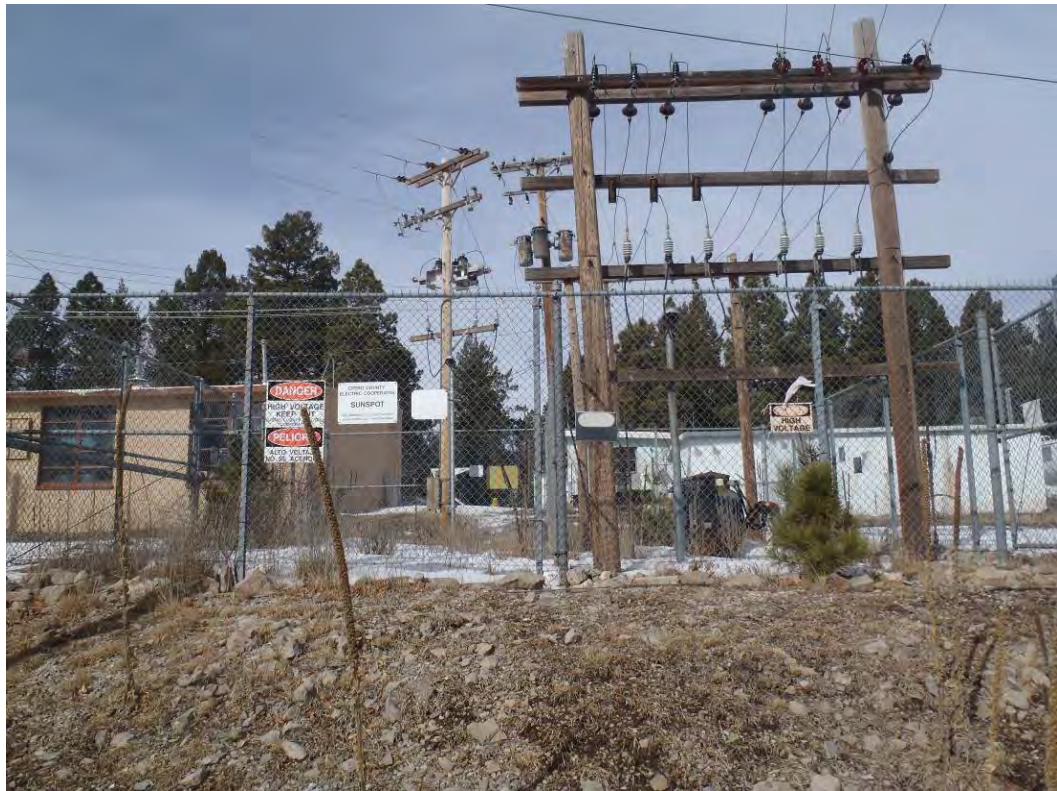
Photo 14: Transformers next to generator building facing west
