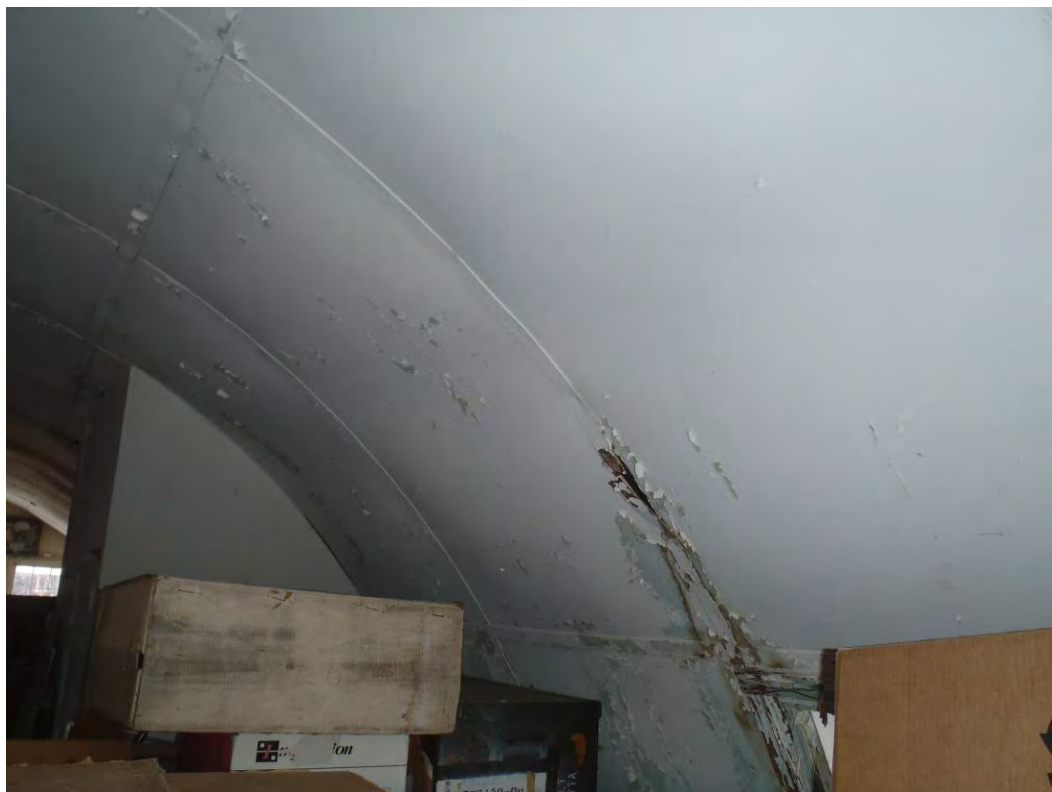
Photo 68: Paint peeling inside storage Quonset hut
