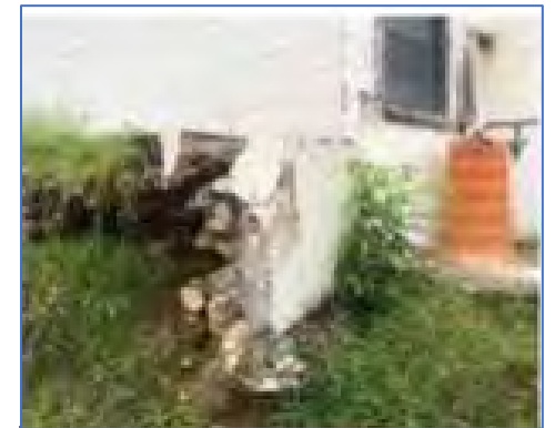
Cable Car Building (Building 5) Damaged Retaining Wall
