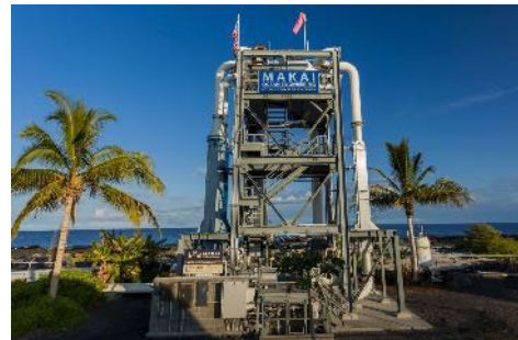
Ocean Thermal Energy Conversion
