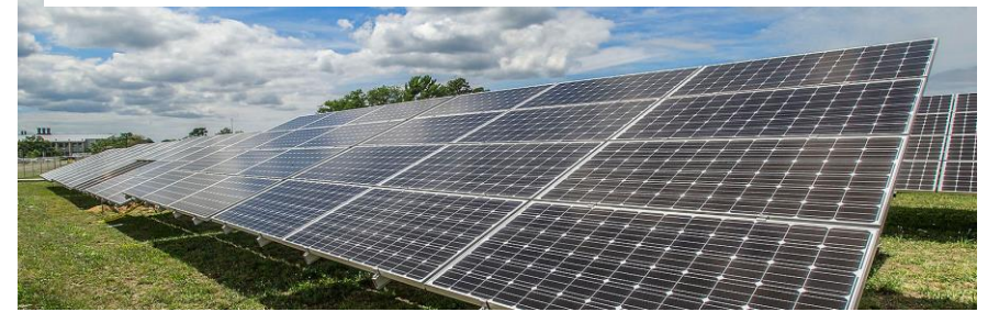
BNL's Northeast Solar Energy Research Center
