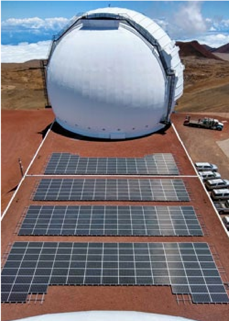
Keck Observatory photovoltaic panels
